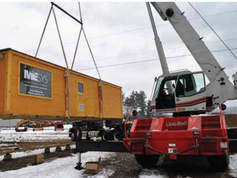
Mt Abram's installation of a containerized pellet system heats the 7,500-foot base lodge, displacing about 12,000 gallons of heating oil annually. COURTESY MT ABRAM
