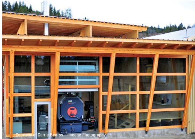
Courtesy of Carrie Bearss – Imedge Photography Custom-built boiler house with wood chip fuel storage bunker and walking floor feed system
